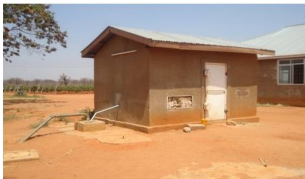
Plate 3: One of the water pumping stations at Chinangali II (Photo by: Author, August 2016)
